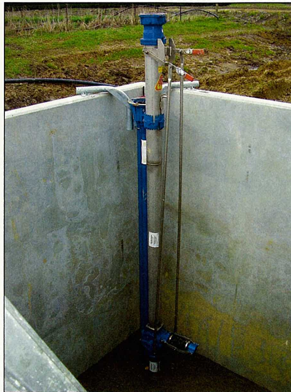
Another deep sump sludge pump installed. Note the mixing nozzle at the bottom. The reverse screw impellor is submerged.
